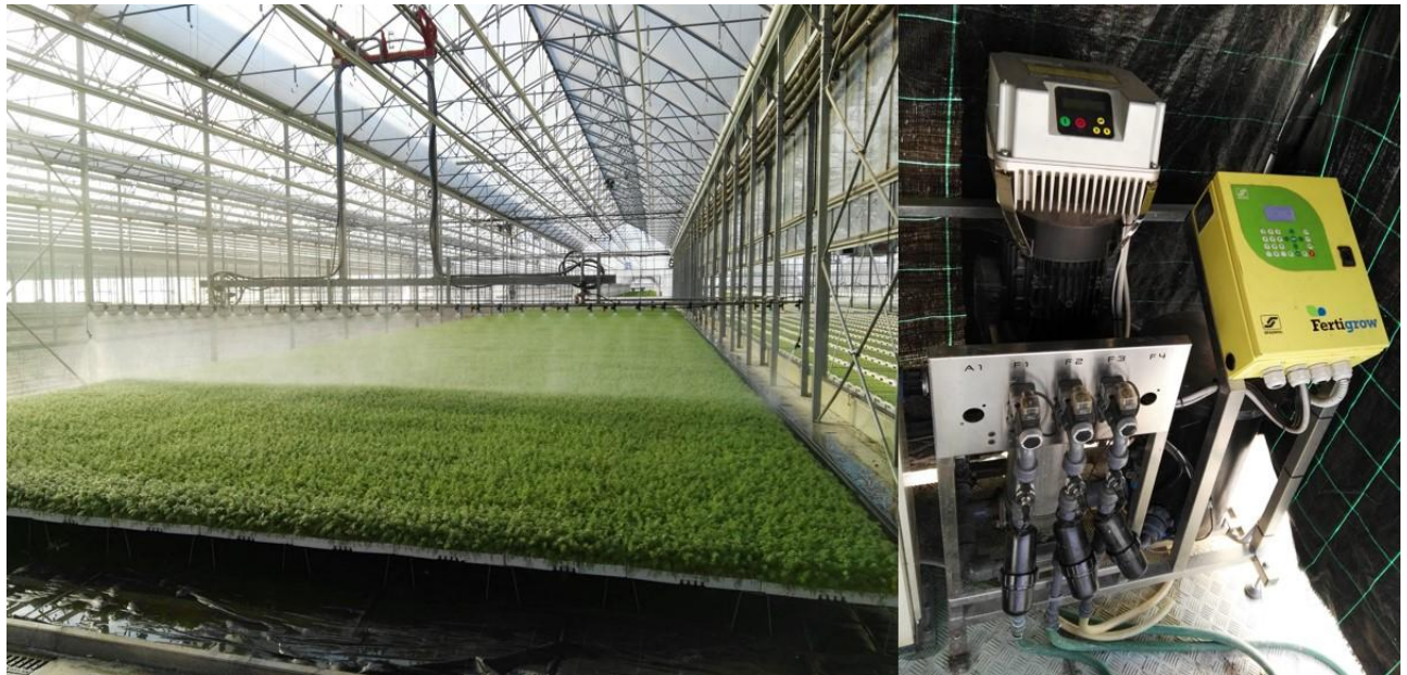
Fig. 5 – spraying equipment in greenhouse and proportional dosing device
