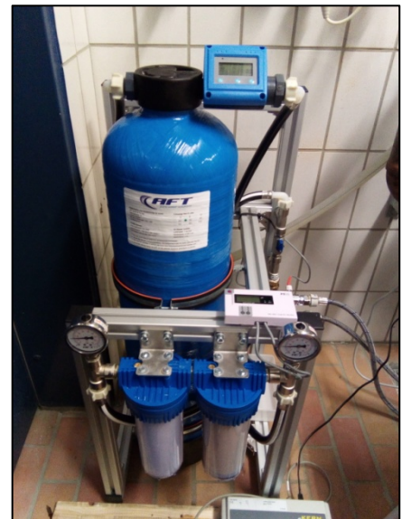
Figure 9: Demineralizer AFT VE-Station 100 Mono (final solution)
